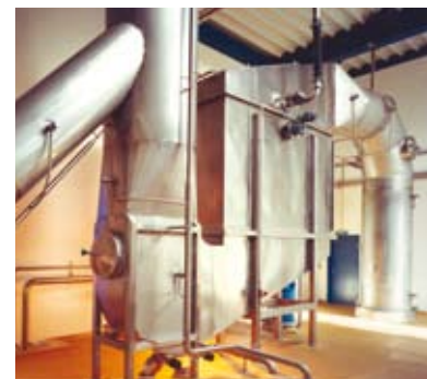
Process thermal heat recuperator unit and ducting equipped with CIP nozzles
