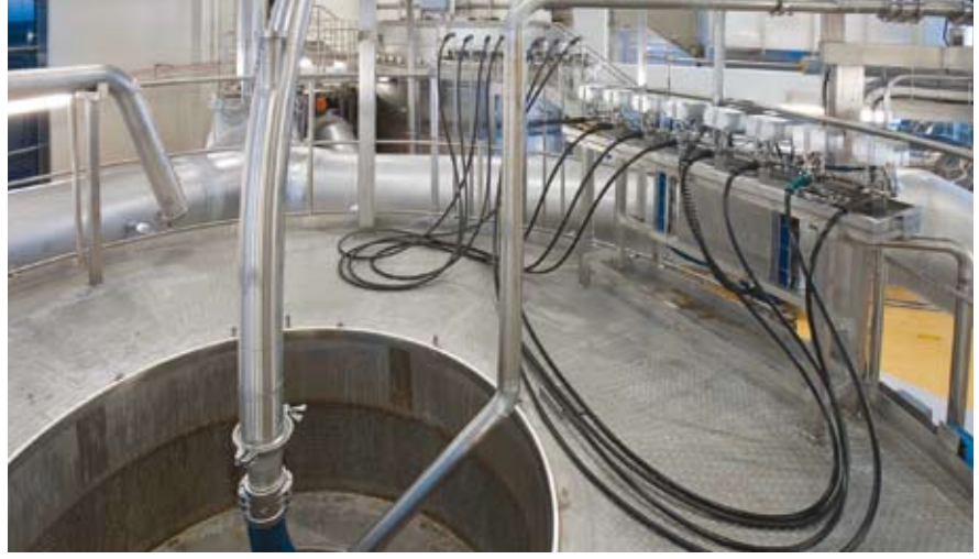
Spray drying chamber in CIP mode. Atomizer nozzles removed from atomization zone. A CIP turbine cleans surface of inner chamber walls
