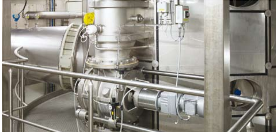
CIP nozzles installed to clean the integrated fluid bed and the spray dryer
