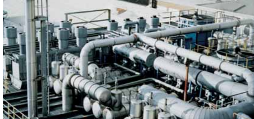
Four Dry Condensing Units on the roof at Walter Rau, Neuss, Germany
