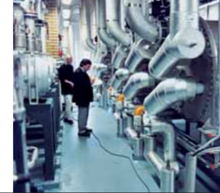
Two Dry Condensing Units at AAK, Karlshamn, Sweden
