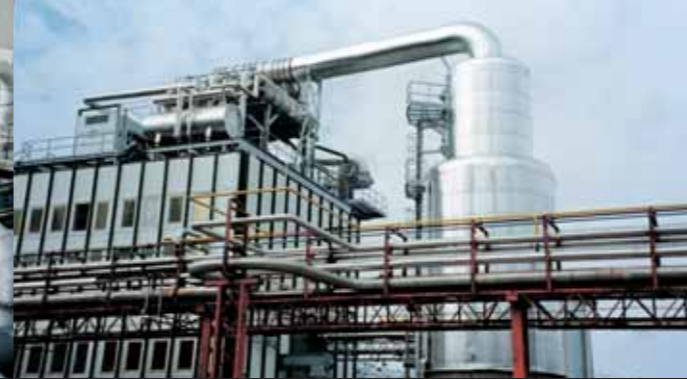
Dry Condensing Unit on the roof at Cereol, Martfü, Hungary
