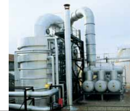
Dry Condensing Unit at Cereol, Bordeaux, France
