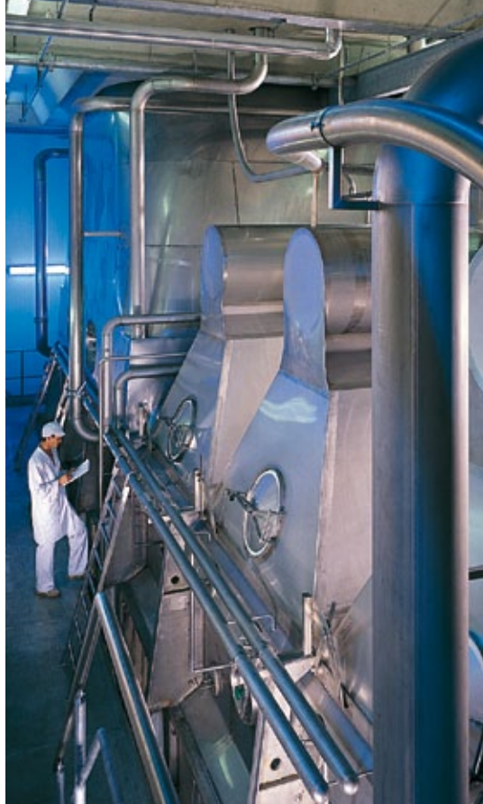
Final drying sections with venturi design for air-flow
