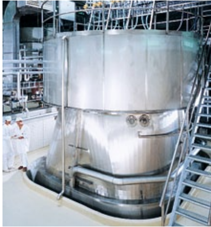
Top of drying chamber showing air disperser
