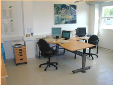
Process control room
