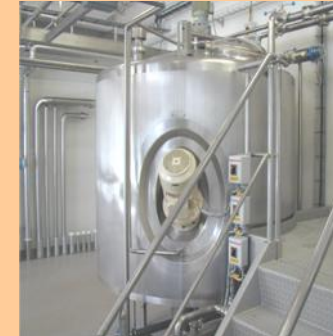
Wet mix tank
