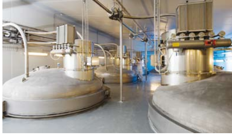
Top of the powder silos and the air filters for the conveying air. The silos can be CIP cleaned
