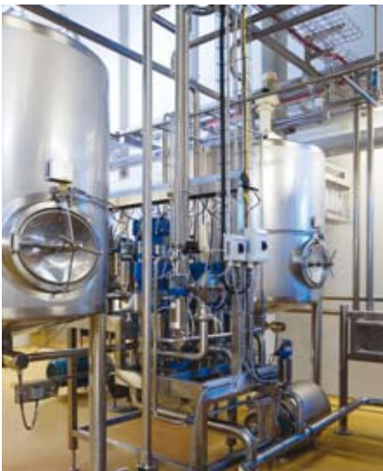
Two feed tanks fully enclosed with CIP spray balls and automatic changeover from one to the other. One is in use while the other is being cleaned
