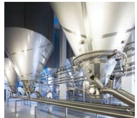
For conveying of powder to the bagging off line or retail packing, the bottom of the powder silos are equipped with pipework
