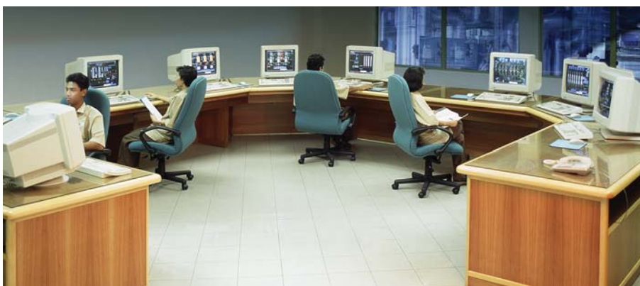
Process control room
