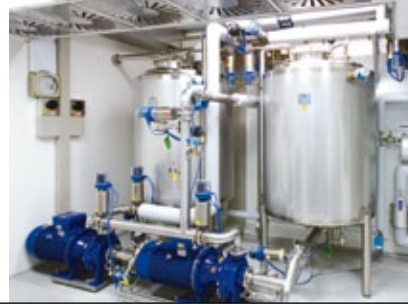
PSD-4 CIP (Clean in Place) tanks.
