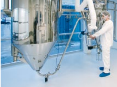
PSD-1 spray dryer in clean room.
