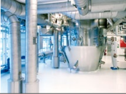
PSD-4 chamber and HVAC ducts.
