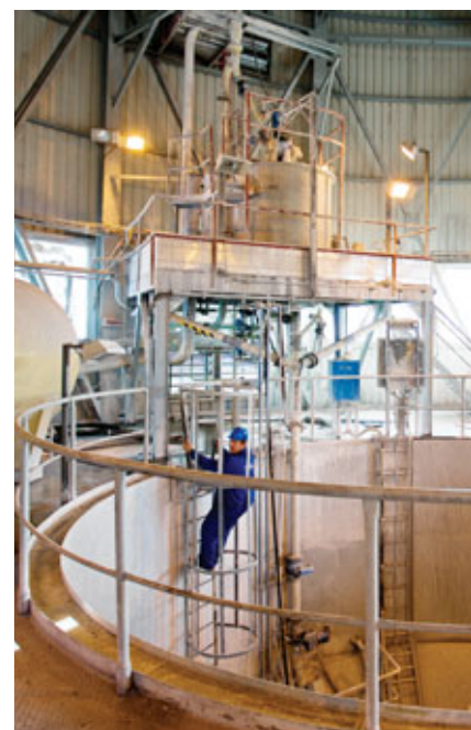
Absorber penthouse with absorbent supply arrangement and spare rotary atomizer.
