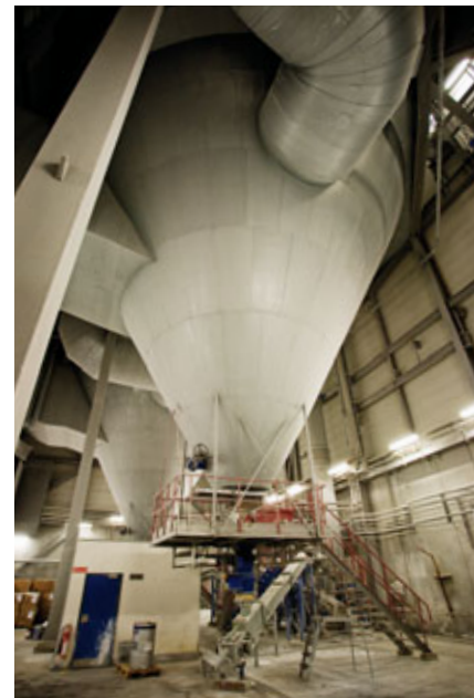
Bottom of SDA with flue gas inlet and outlet duct and product discharge.
