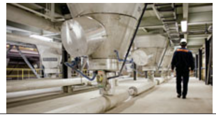
Right: The dry free-flowing product from the SDA process can easily be handled in a pneumatic transport system.
